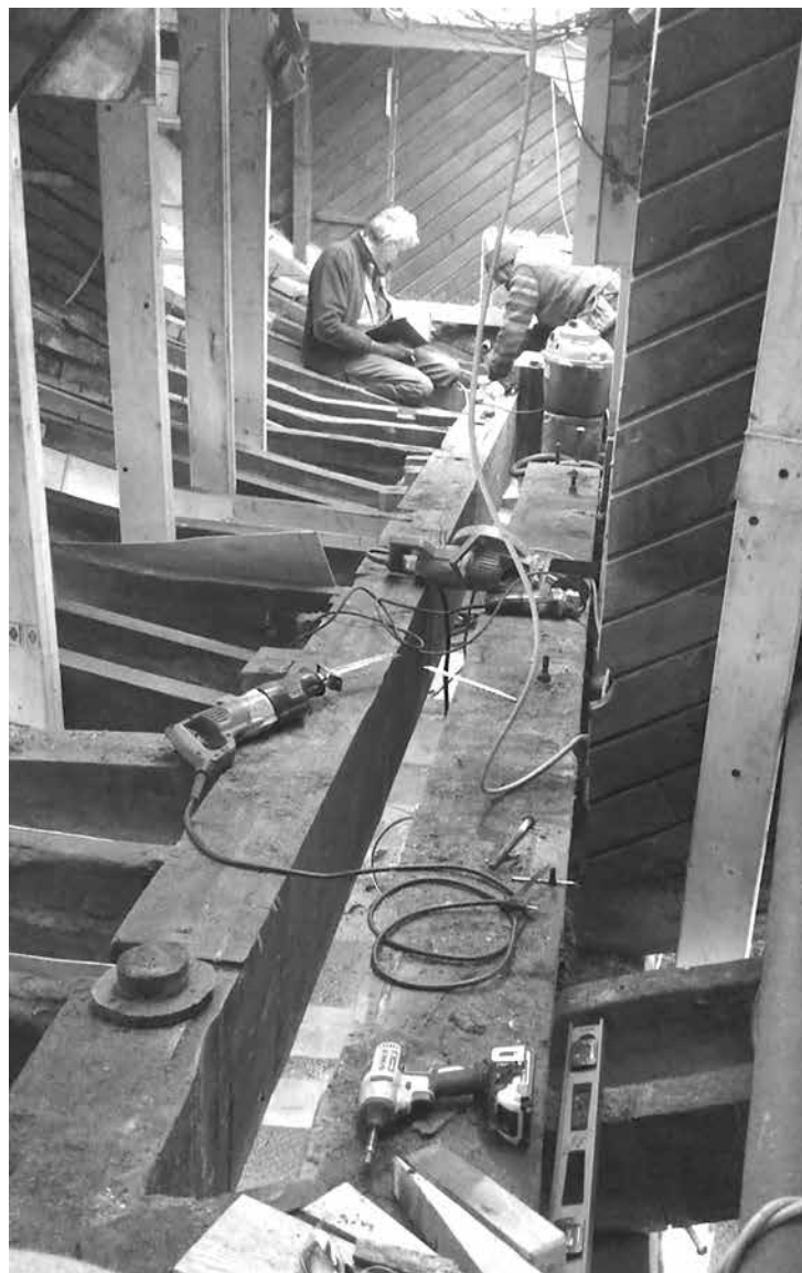
Jim Kricker and Wayne Ford work inside the "Clearwater's" midship during its massive 2015/2016 rebuild and restoration at the Hudson River Maritime Museum
